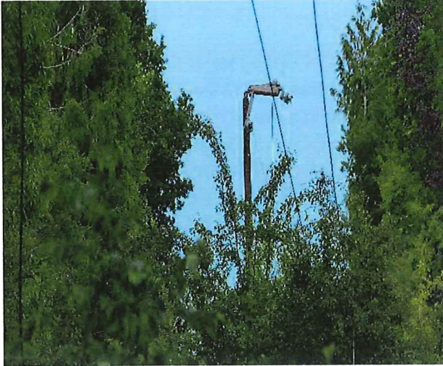
One of the pylones 20 KV destroyed after a falling down of tree on the electricals lines
